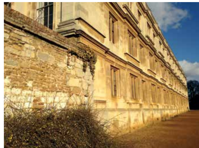
Clare College Old Court, south range, 1640-42, built of Ketton Limestone, the most commonly used stone in Cambridge.
