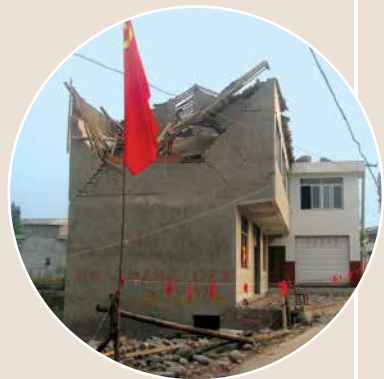
Damage to rural houses after an earthquake
